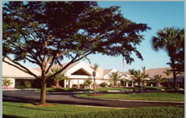
Stonebridge Country Club – This project involved extensive renovations, new additions to the kitchen and card rooms and construction of a new fitness center.
